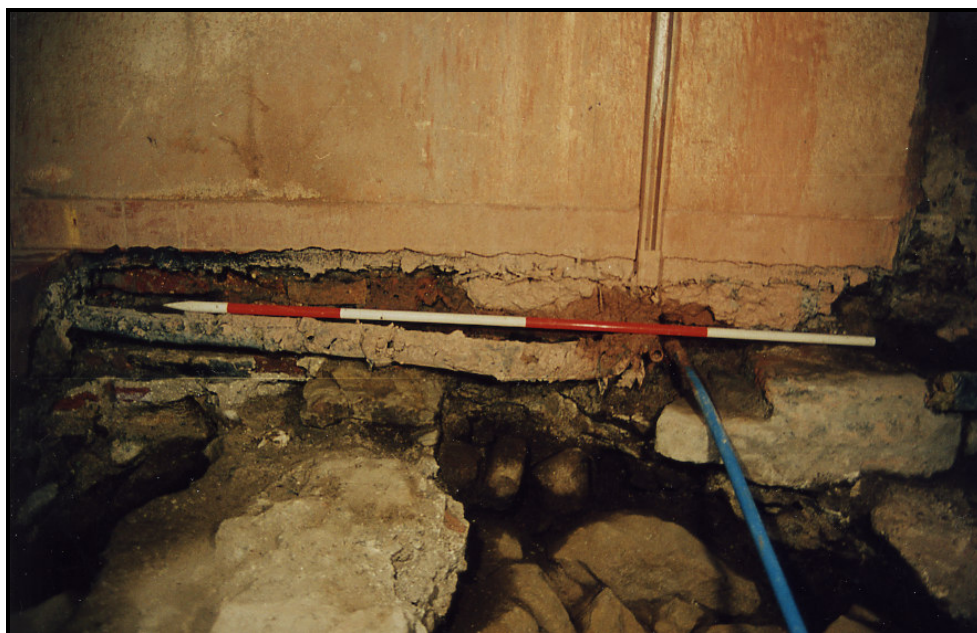
Plate 3: View of the visible traces of the plinth at the base of the keep wall.
