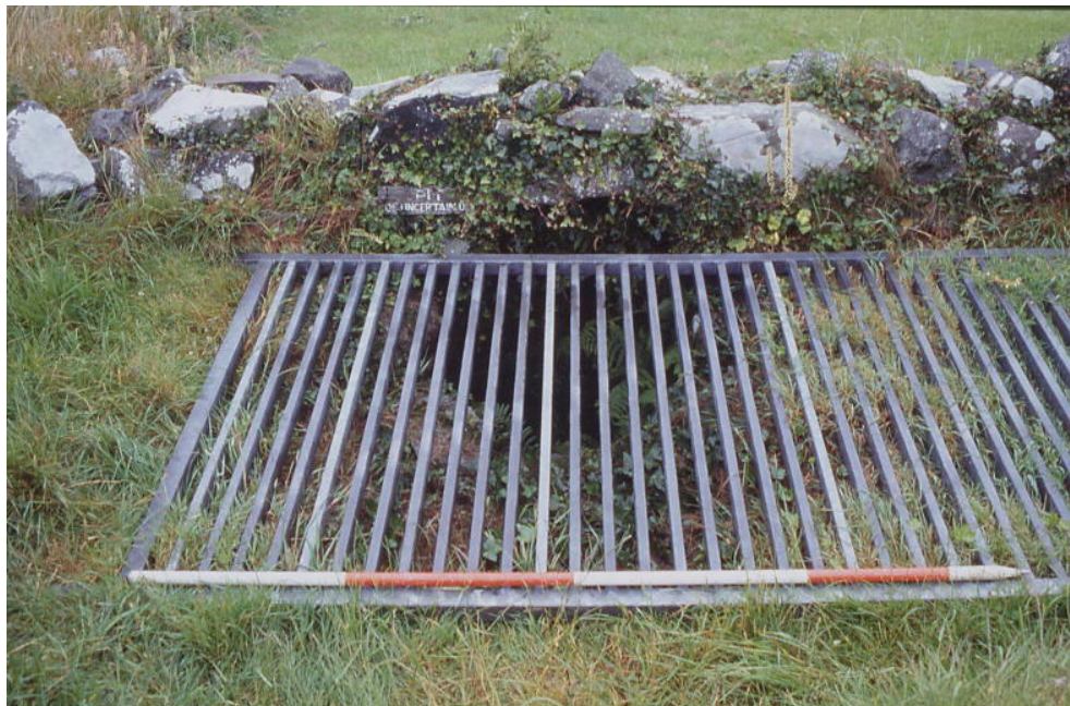
Plate Two: The exposed pit prior to the removal of the old safety grill looking northwest.
