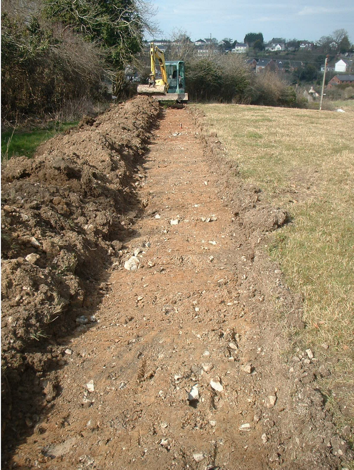
Photo 1: Excavation of Tr. 1 showing utilization of toothless “sheugh” bucket and surface of subsoil (Context 102).
