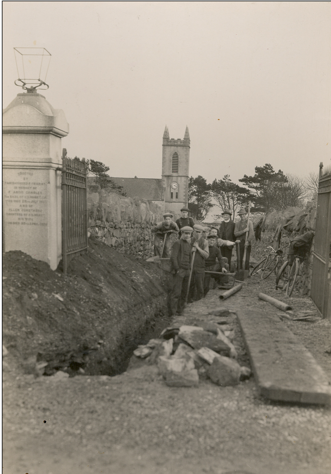
Plate Two: Photograph in possession of Kilhorne Church showing excavation of trench to accommodate water pipe (1932). The photograph depicts Sammy Heaney, Willie Cousins, Rev. T.H.Lyons, Archie Gordon (rear) and John Reidy, Alex Orr, James Gibson, Jim Annett, Ernie Mooney, Hugh Bell (front row). Photograph kindly supplied by the Reverend William Press.
