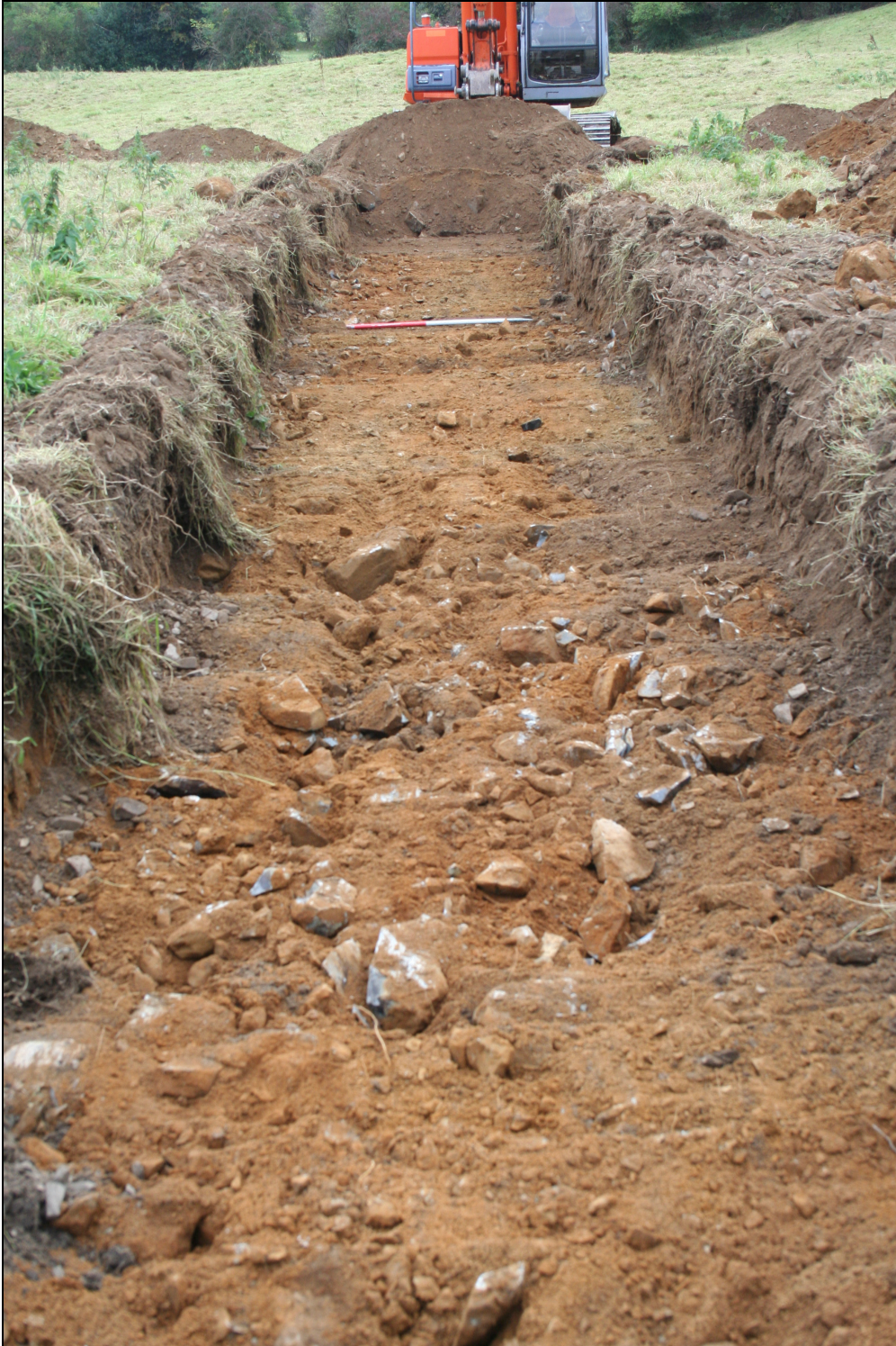
Plate 5 Excavation of Trench C, looking SE, showing topsoil (Context No. 301) directly overlying glacial sub soil (Context No. 302)
