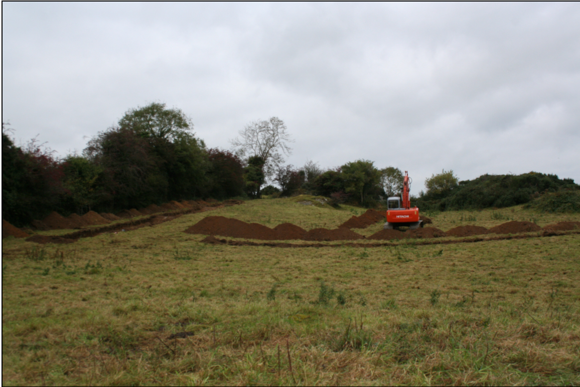
Plate 1 General shot of proposed development site looking NW during excavation of Trench C. Note the entrance 'ramp' to the left of shot along which Trench A was excavated.
