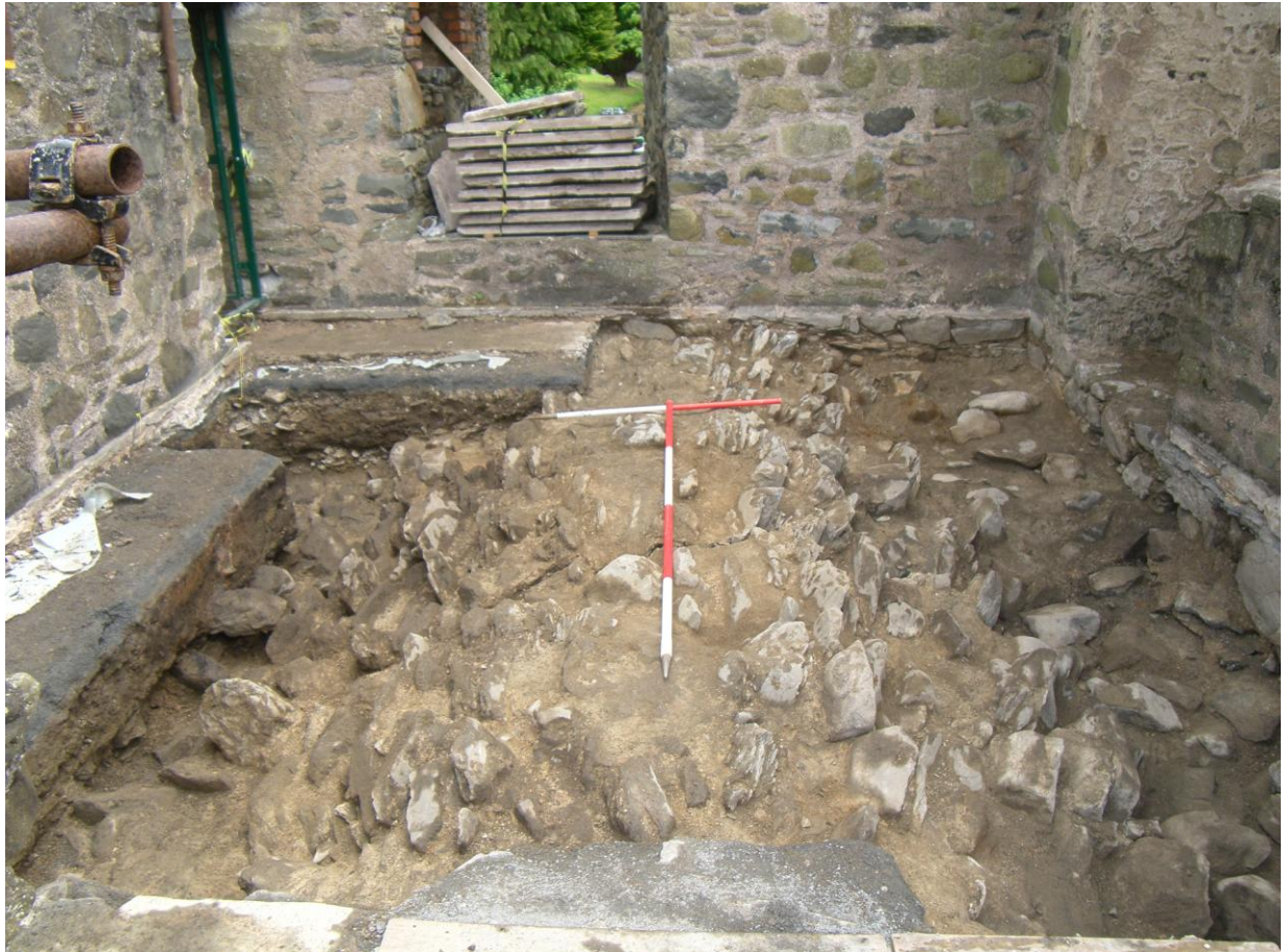
Plate 3. Quoile Castle, Co. Down. The southern chamber. Exterior surface of the first floor vault fully exposed after excavation. The crack in the vault roof is visible, running left to right across the middle of the photograph. From the west.
