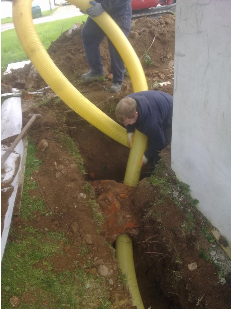
Plate 6: Installation of the drainage pipe beneath the foundations of the red brick wall (Context No. 202) looking east.
